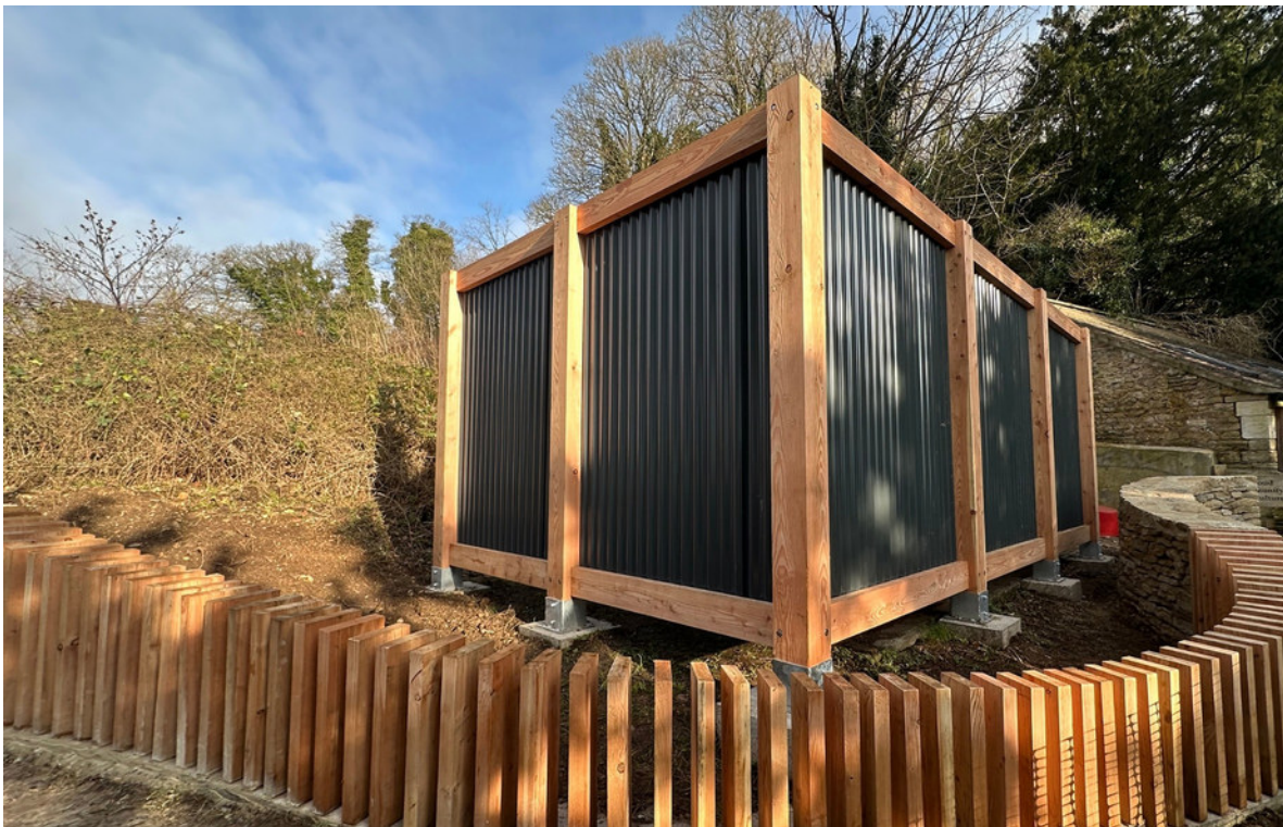
Images showing resident artist Kate McMahon-Parkes, Malcolm McMahon and stone waller Sam Usbourne building the Loom Wall which screens SCA's chiller unit and creates an entrance to Hawkwood.
